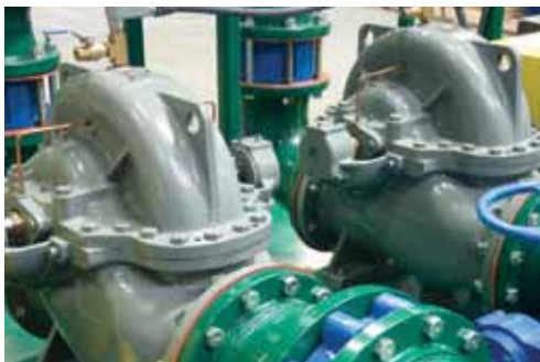
Water Feature Pump Station
