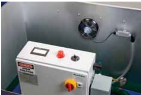
Interior of Low Profile Pump Station (LP)
